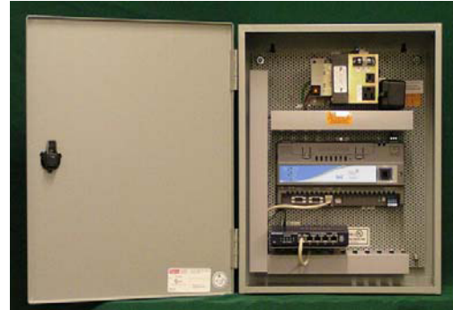
PAGx00001FC0 NAE Standard Control Panel Assembly Mounted in a 16 in. x 20 in. Enclosure
